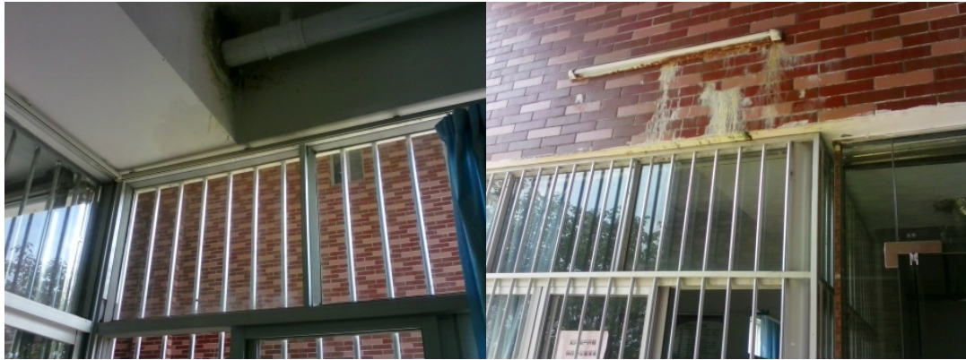
宿管科漏水实情
